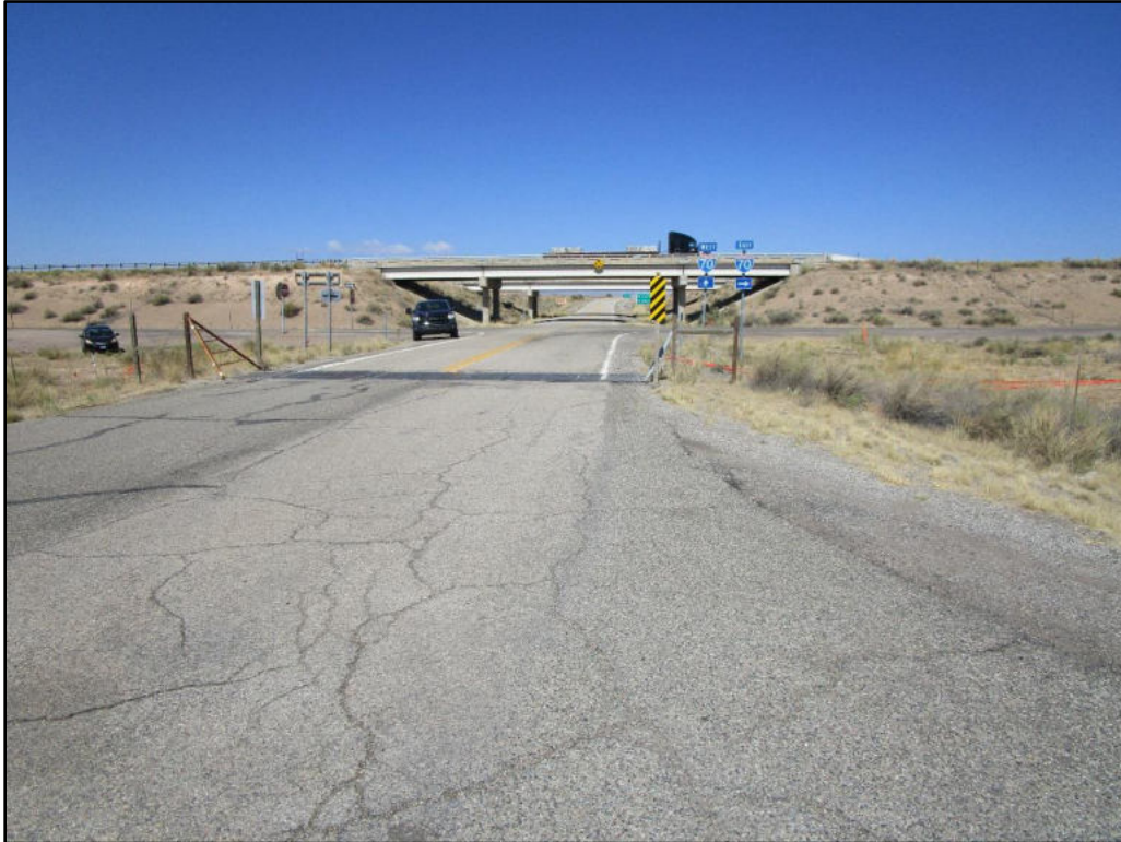
Site 42GR2305. Site overview from south end of road from SR 128 (Crescent to Cisco East Rd); view to the north showing I-70.
